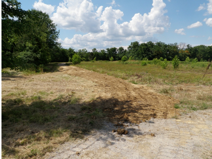
Shor Park Wetland Restoration and Storm Water Demonstration Project in progress, Union Twp, Clermont County
